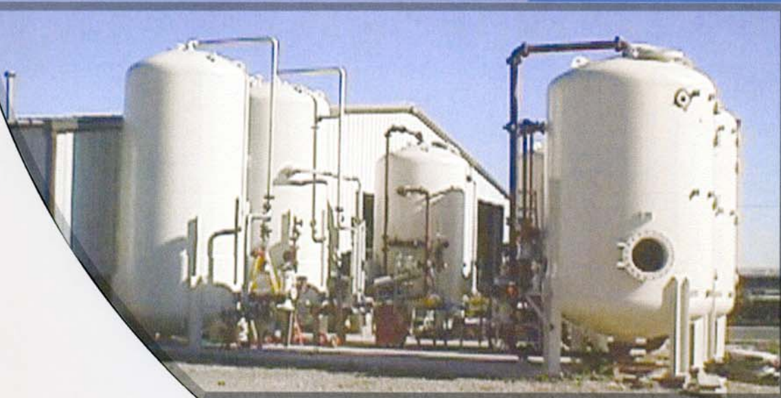
High Purity Water Systems
